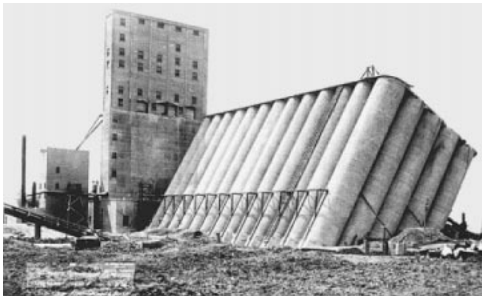
Transcona Grain Elevator after failure.
