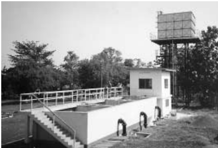
Filter units at Yendi treatment plant, with the backwashing tank in the background.
