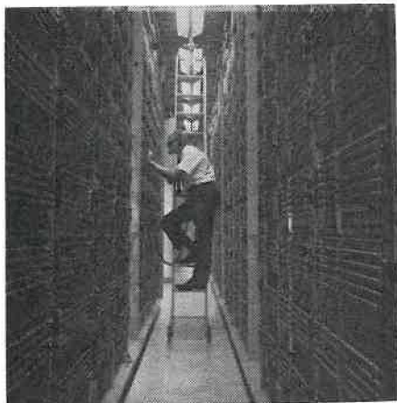
Cross Bar Switches on 4-A Trunk Line Frames
